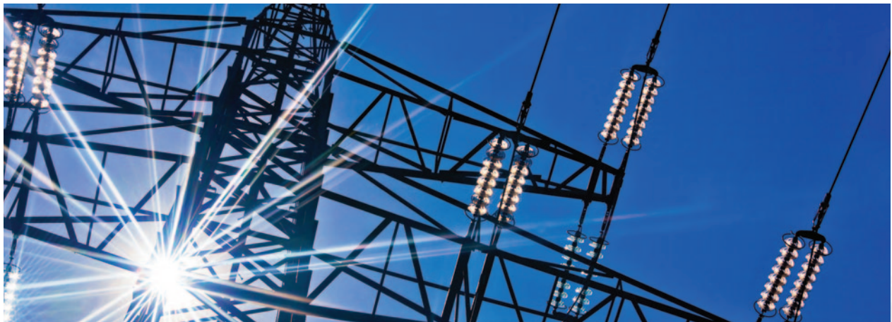
Electricity pylon. © Lisa S
